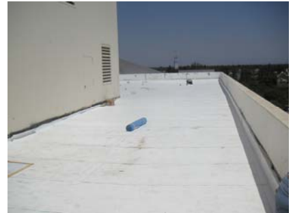
Waterproof Membrane on CLC
