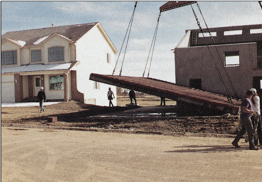
The thickest panels, used for the roof, have an R value of 42. Here a large roof panel with the tiles already installed is being lifted from the casting bed.
