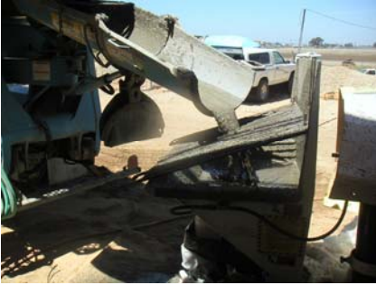
Ready Mix Filling Pump Hopper
