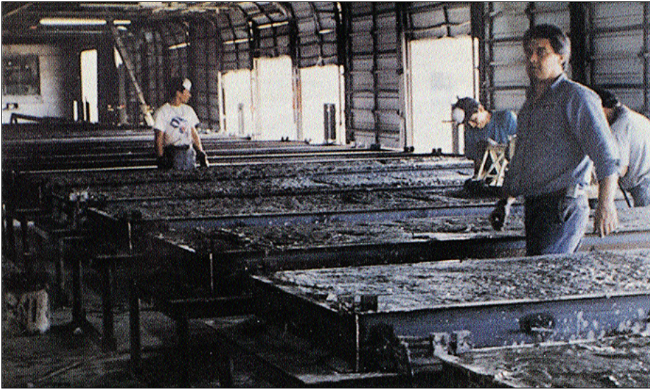
Panel molds are filled to about 50% capacity. The foam concrete then expands over four hours to fill the molds to capacity.
